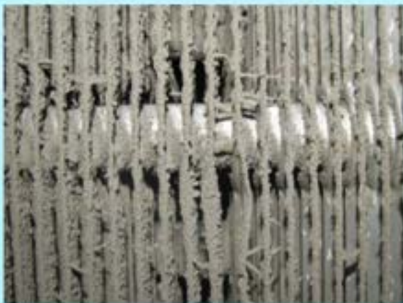
Typical AC system coil before cleaning
